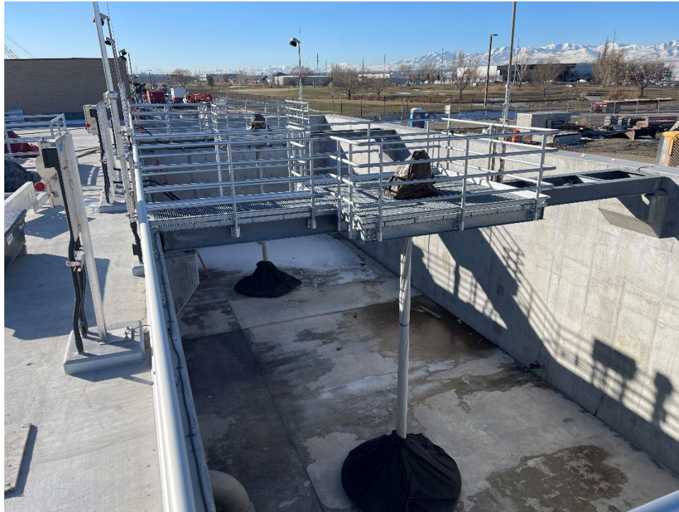
View looking S/W inside the RAS Selector
