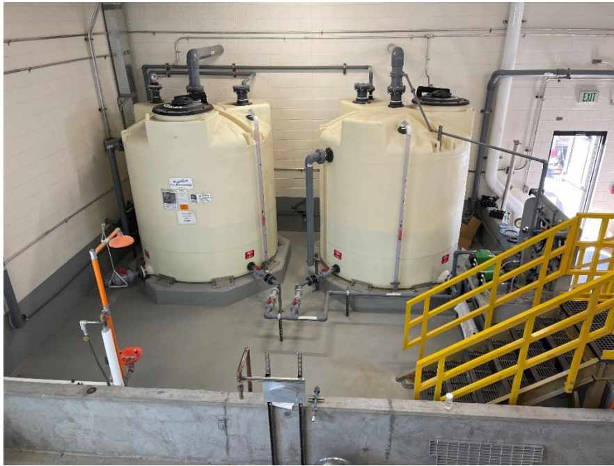
View of the 3W Sodium Hypochlorite tanks looking West
