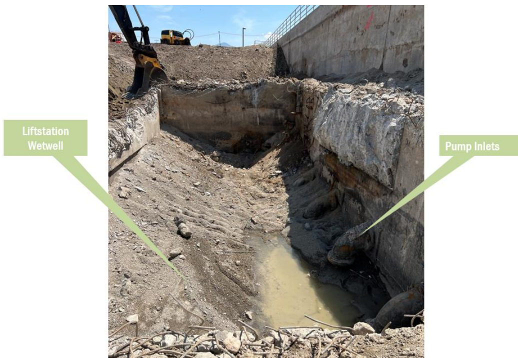
Influent Pump Station Wetwell of SLC Suburban District No.1 Plant
