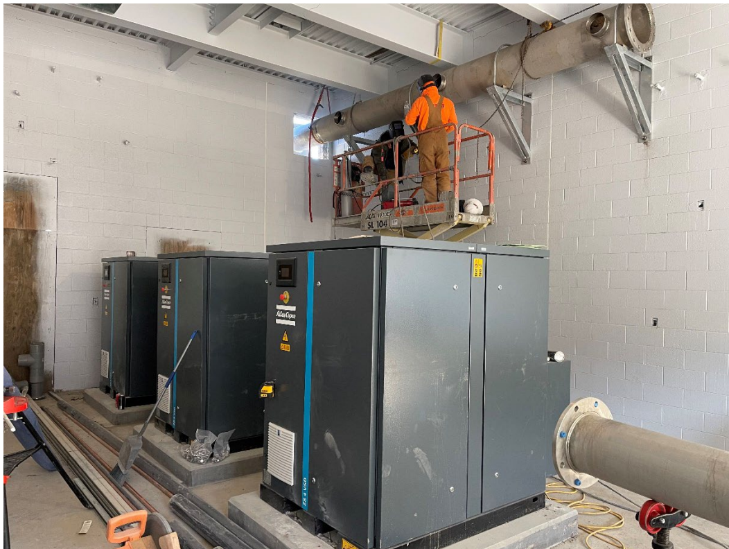
View looking N/W at the Blowers in the SSN Building
