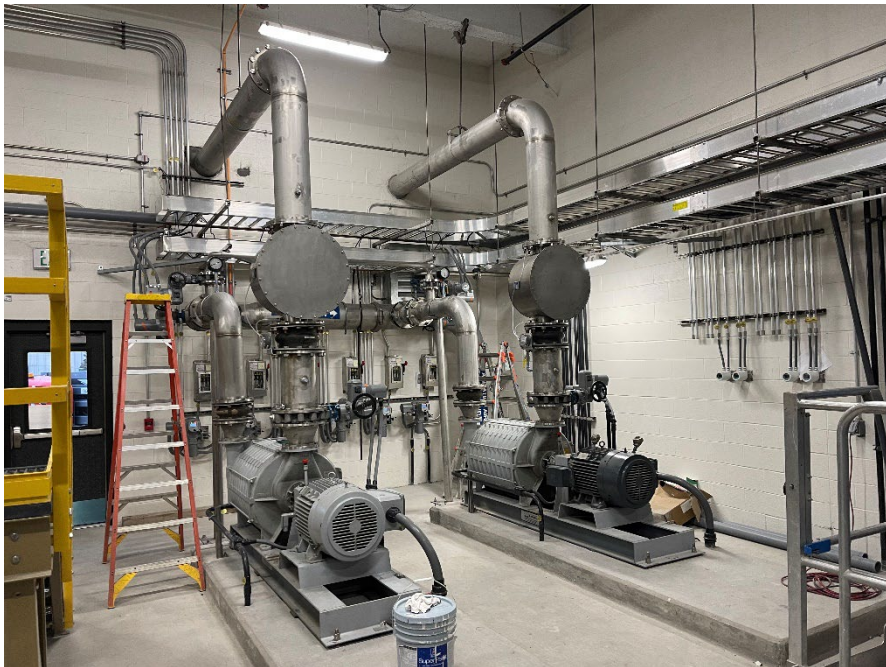
View of Relocated Post Aeration Blowers
